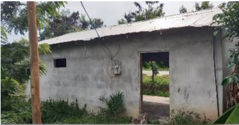
Figure 9-2: Electricity connection to an 'option' structure
