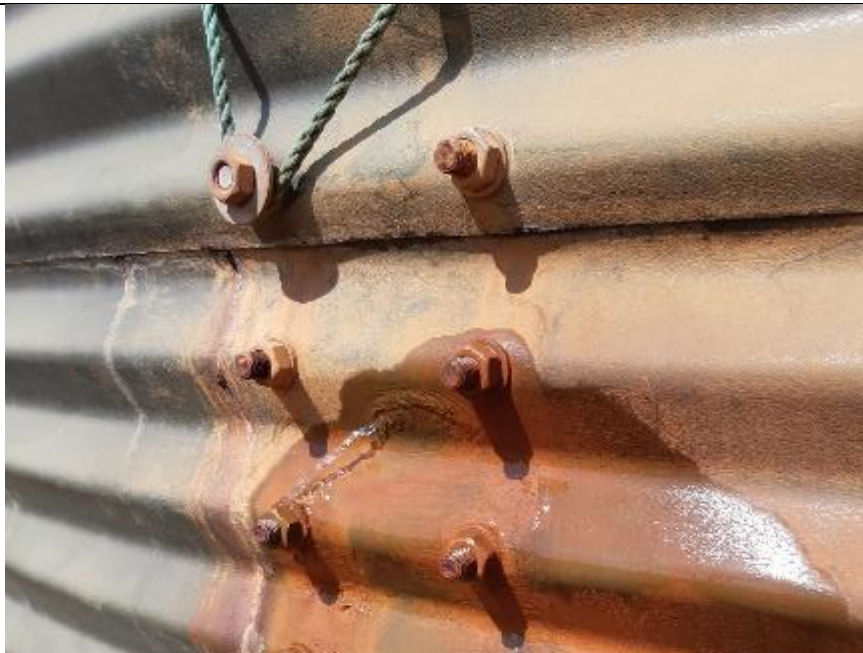
Photo 13. Leaking fire water storage tank at the Pilot Camp
