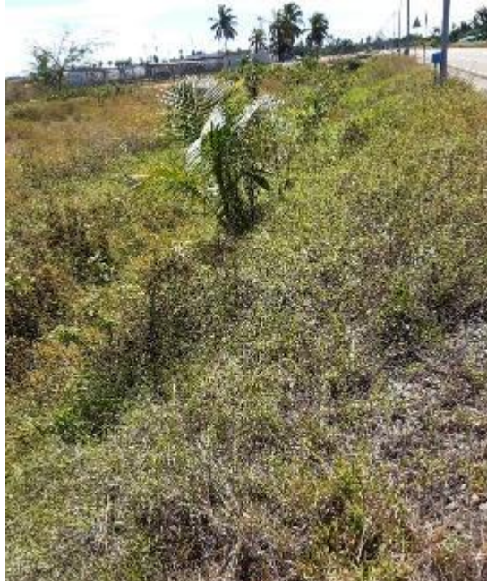
Photo 3. Drainage channels with established vegetation reducing sediment in discharge of surface water from site
