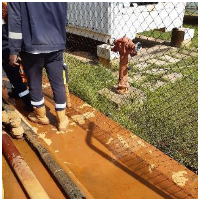
Photo 14. Pooling water resulting from leaking firewater storage tank
