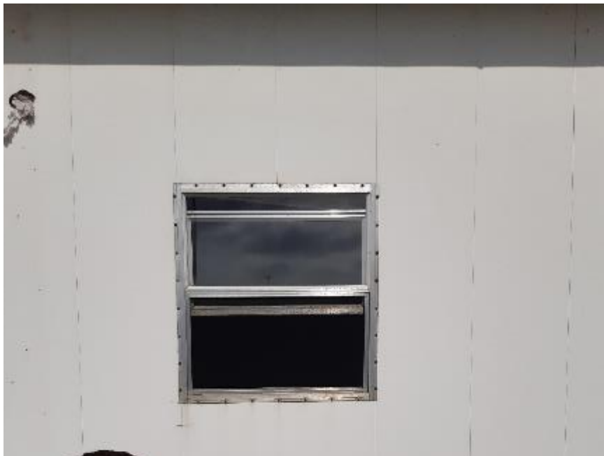
Photo 18. Windows left open in air-conditioned rooms
