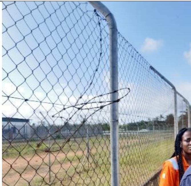
Photo 11. Rusted and loose barbed wire at head height around the pilot camp presents a hazard to residents, particularly at night when visibility is poor
