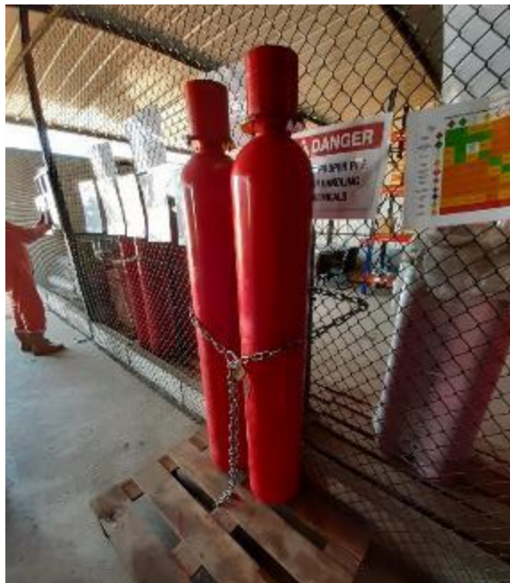
Photo 8. Gas cylinders sitting on a pallet and secured to wire fence as a temporary measure -risk of toppling
